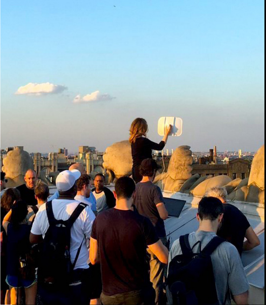
NYC Mesh Member leads an install training workshop with a Litebeam router.
